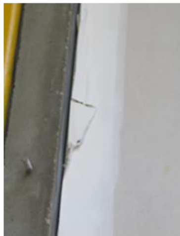
5. Screw breaking on panel edge
