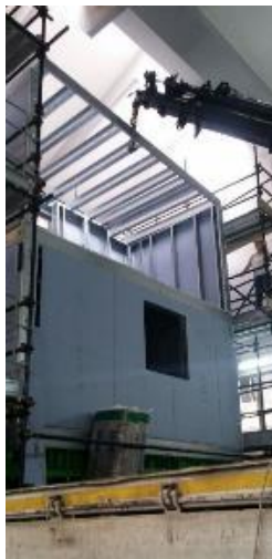
Walls and floors lifting
