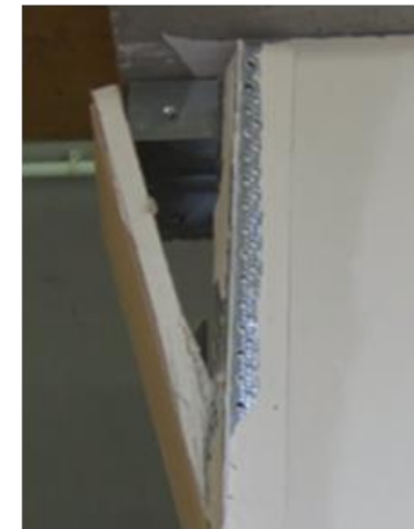
6. Stud to track fixing failure
