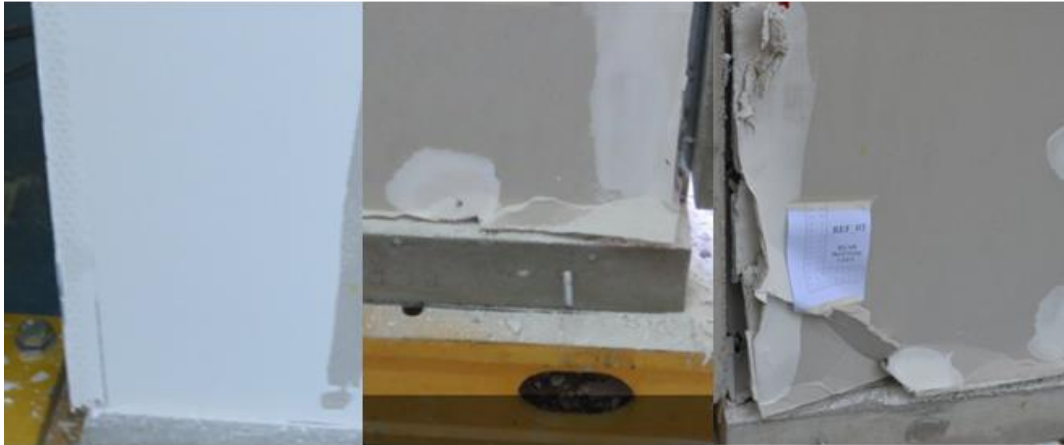
1. Rupture, crushing or spalling of panel portions
