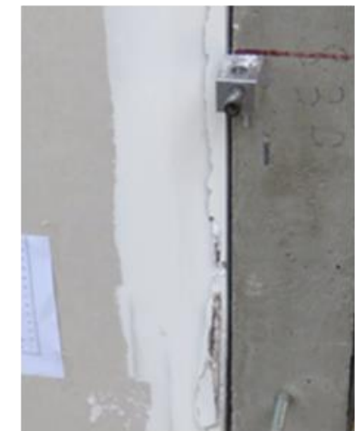
7. Gap opening between panel and structural elements
