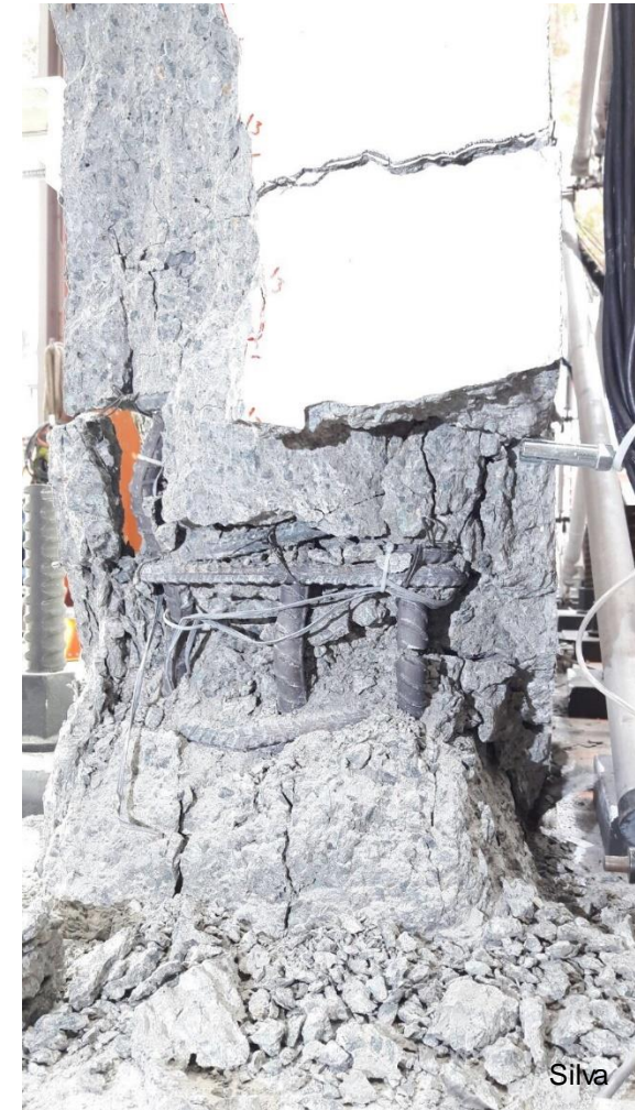
Flexural wall toe failure
